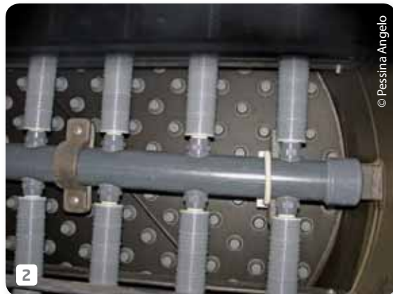
2 Interior view of one of the exchangers coated for SESPI Srl by Pessina Angelo.
